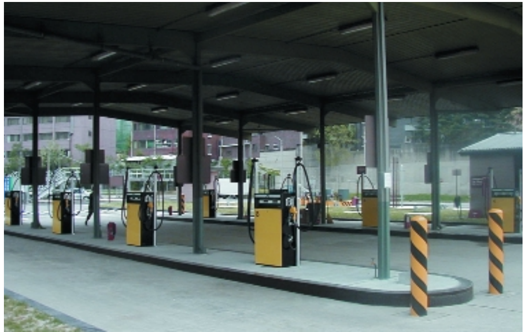
The Yongsan TMP after its upgrade. The project was the latest milestone in a comprehensive Defense Energy Support Center upgrade of bulk petroleum and TMP fuel facilities in Korea.
