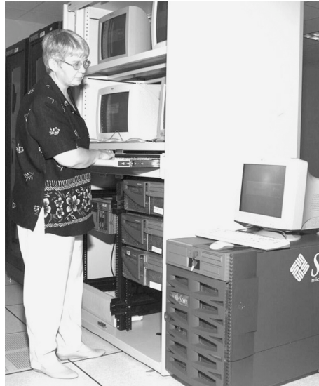
Peggy Norris, a technical data specialist who is one of the JEDMICS functional system administrators, checks the JEDMICS database at DSCC. The system stores about 5.5 million technical drawings used by contractors who supply parts and equipment to the warfighter. (Photo by David Benzing)
