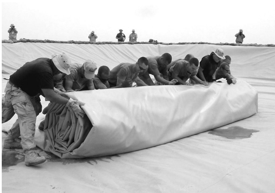
Fuel specialists at Tallil Air Base in southern Iraq, unroll the final 210,000 gallon fuel bladder. The new bladder allows the airmen to fuel aircraft and vehicles used by the Air Force, Army and Marines. (U.S. Air Force photo by Maj. Jon Anderson)
