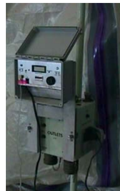
Pressure gauge with differential pressure alarms
