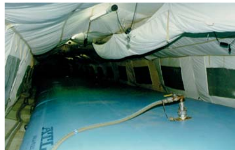
CB hardened water distribution system
