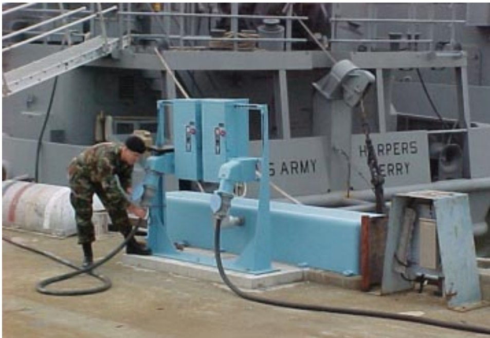
(left) Maj. Steven Strem checks relocated pier electrical power near Army landing craft.
