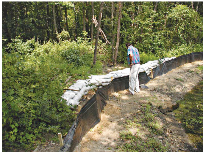
Maryland DNR fishery biologist Bob Lunsford examines a berm of sandbags and silt fences strategically placed to prevent pond water overflow or overland fish migration from Crofton Pond to the Little Patuxent River. Photo by Walter R. Courtenay, Jr., USGS.
