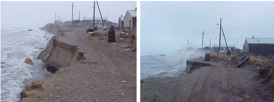
Figure 20: Coastal Storm on October 8, 2002 – Coastal Road in Shishmaref (located on Sarichef Island, Chukchi Sea), at around 12:30pm (l) and 2:30pm (r) (Source: Weyiouanna presentation)
