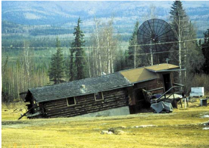
Figure 18: Melting Permafrost Severely Impacts Buildings (Source: Hinzman presentation)
