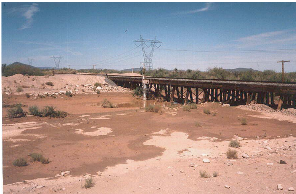
Figure 17. View looking upstream at gaging station from left bank, Centennial Wash at Southern Pacific Railroad Bridge near Arlington, Arizona.
