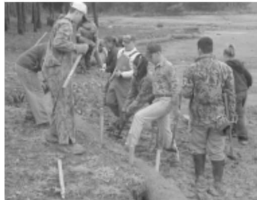
Following the example set by the Little Bear Millennium Project, a group of high-school students recently worked to install some 300 feet of natural materials designed to stabilize soils along the shores of Cedar Creek Reservoir.
