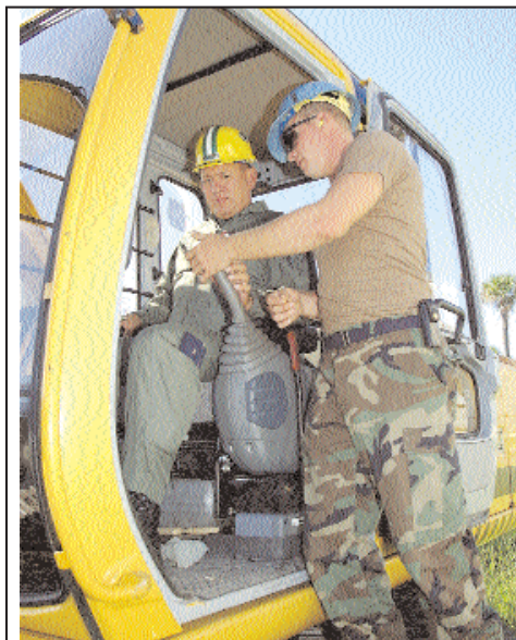
Senior Airman Randall Terry, 45th Civil Engineer Squadron, right, shows Brig. Gen. Greg Pavlovich, 45th Space Wing commander, the finer points of running an excavator before taking down the last section of the HESCO barrier on State Road A1A. All four lanes opened Sept. 13. (Photo by Jim Laviska)
