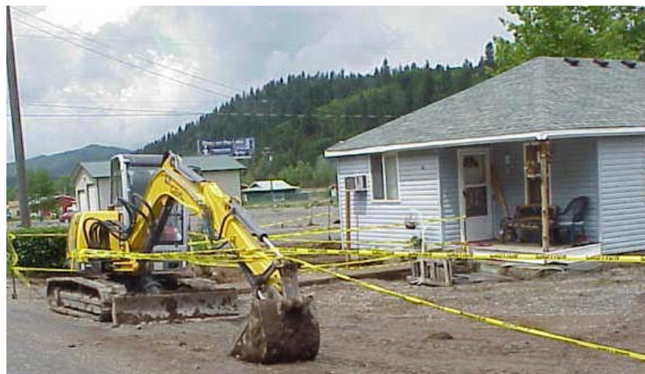
Backhoe preparing to remove contaminated soil from yard in Osburn, Idaho. Yellow tape is used to keep people out of the excavation area during cleanup.
