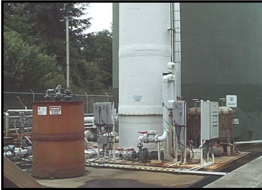
Operable Unit 1, Area 6. View of Area 6 groundwater extraction, treatment, and recharge system (treatment components, stripper tower [white], holding tank [green] and associated pumps/piping).
