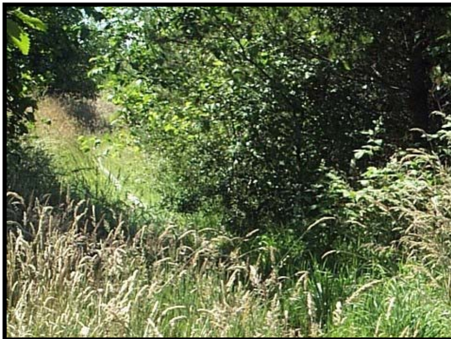
Operable Unit 1, Area 6. View of Area 6 groundwater extraction, treatment, and recharge system (grassed swale recharge area). Note the white perforated poly-vinyl chloride (PVC) discharge line.
