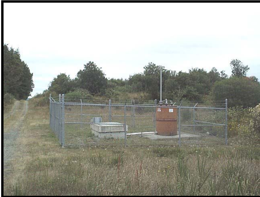
Operable Unit 1, Area 6. View of Area 6 groundwater extraction, treatment, and recharge system (extraction components at location of a production well).
