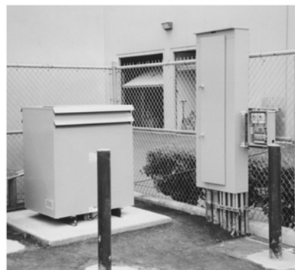
New Electrical Panel, Timer Control and Step-Down Transformer
