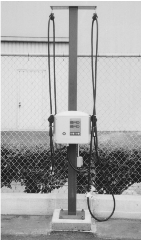
Pedestal-Mounted Power Control Station (PCS) Charges Two ECRVs
