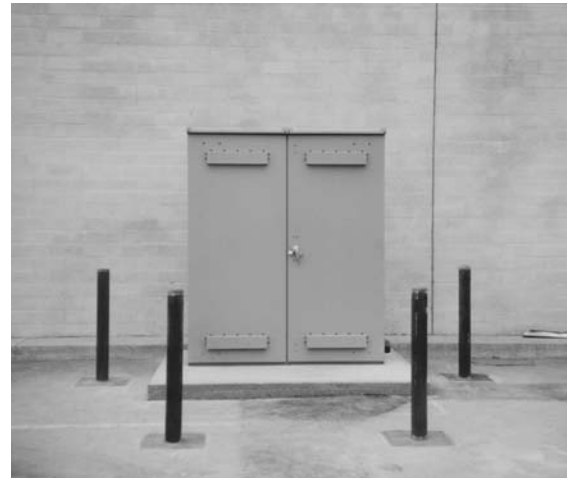
New Service Entrance Section with Meter
