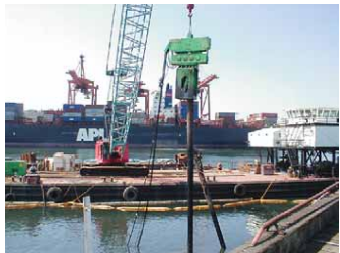
Cleanup at the Harbor Island Superfund site includes removing about 8,000 creosoted piles.
