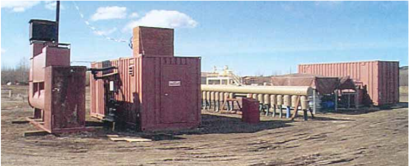
Work at Fort Wainwright has stimulated the local economy, as local contractors are doing the bulk of cleanup.
