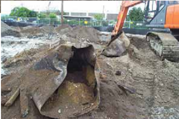
Prior to cleanup, soils at Frontier Hard Chrome were stained with contamination.
