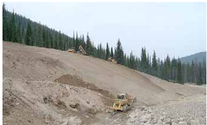
EPA consulted formally with the Kootenai Tribe and the Canadian government to complete a rapid cleanup of Continental Mine.
