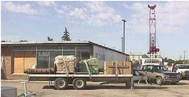
The results of a rapid investigation at Franke's Laundromat are helping EPA and others determine next steps.
