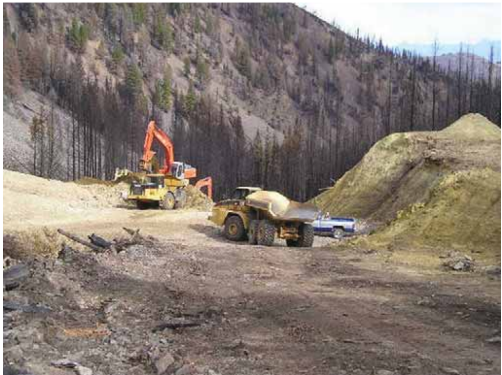
A fast cleanup at the Harmony Mine protects downstream waters from copper contamination.
