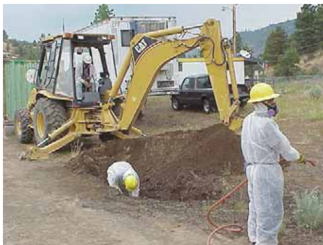
EPA takes fast action to remove asbestos from the North Ridge Estates neighborhood.
