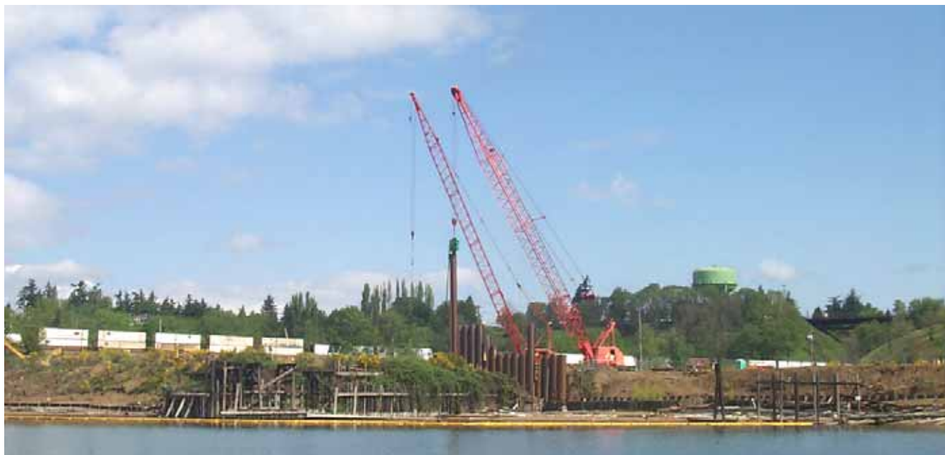
The sub-surface barrier wall at McCormick and Baxter will prevent toxic substances from seeping into the Willamette River.
