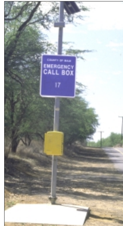
An emergency call box located in a rural area is mounted in an accessible location and can be used with or without speech to provide effective communication.
