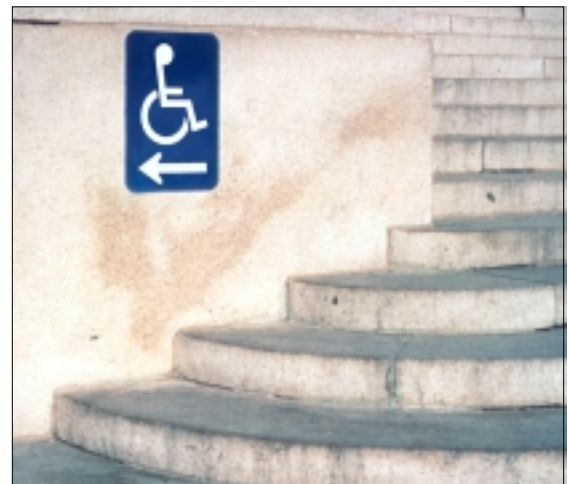
Sign at an inaccessible entrance provides directions to the nearest accessible entrance.
