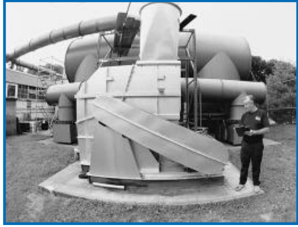
The fan on the RTO is more energy efficient after a VFD was installed.
