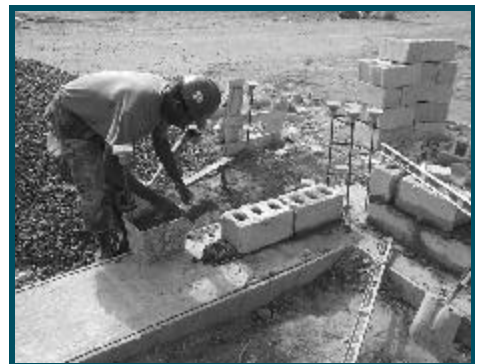
BU3 Larry Hayes places the first course of masonry block for a humanitarian Clinic being constructed in Senegal, Africa.
