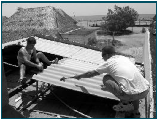
Thanks to prior experience two Marines are able to make short work of a leaking roof the Boquilla High School a few mile from Cartagena, Colombia.
