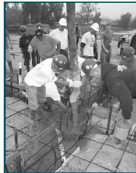
CE1 Alan Reyes (foreground, in white shirt) guides the discharge hose pumping concrete while CE3 Giovanni Perichi (right, with shovel) spreads fresh concrete into the forms.
