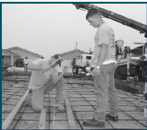
SW2 (SCW) Andrew Palmer (left) and SW3 James Muskevitch prepare forms prior to a concrete pour.
