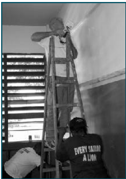
NC1 (SW) Lejeune D. Chute of Myrtle Beach, S.C., holds the ladder as DK3 Christopher Glass of Dallas trims a classroom wall at the municipal School Georg Pfisterer.
