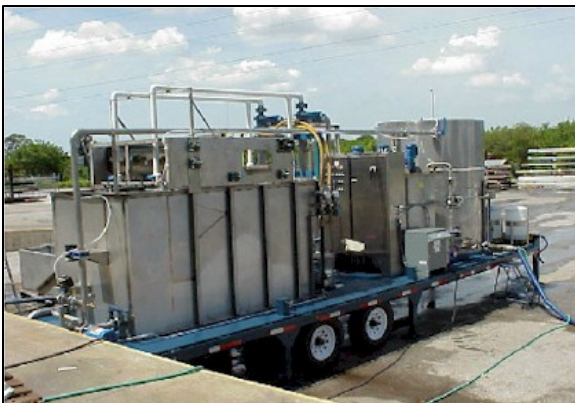
Air Sparged Hydrocyclone System for AFFF removal.
