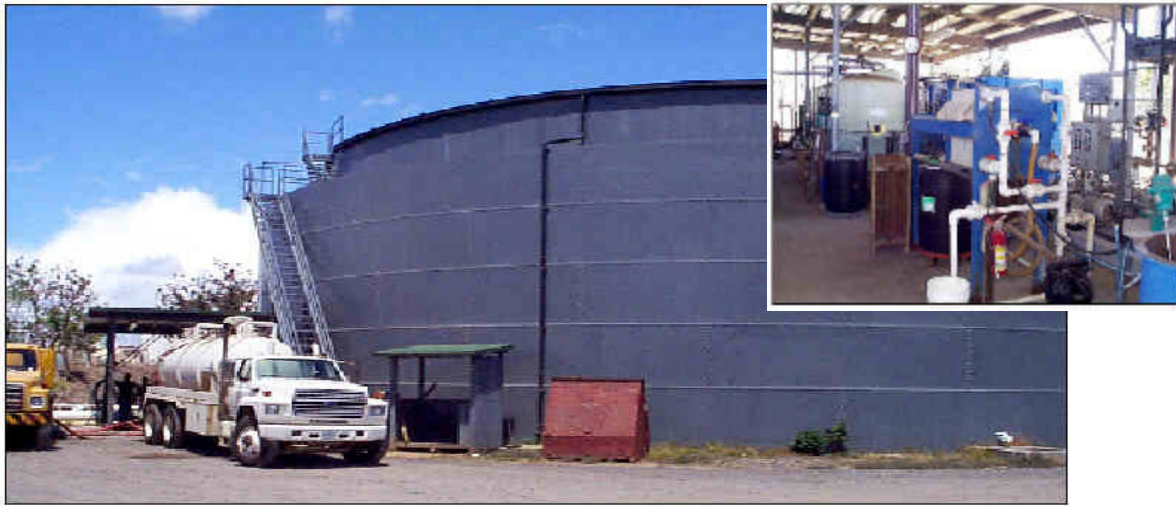
Bilgewater Treatment Facility
