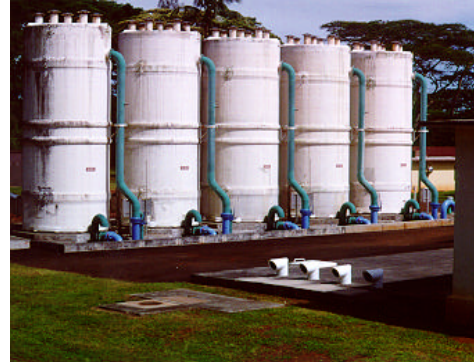
Schofield Barracks Packed Aeration Towers Used for Removal of TCE
