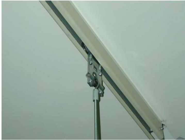
Figure 3.1 – Rail Track in Ceiling
