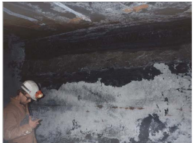
Figure 10.—As a weak seat earth thickens in a southern West Virginia mine roof, it causes roof bolts to miss anchorage in a strong sandstone.
