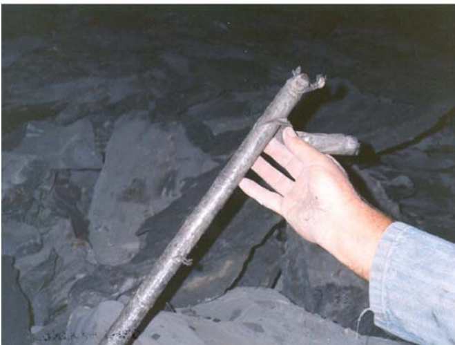
Figure 46.—Two views of "glove-fingered" bolts that provide little mechanical interlock to support strata.
