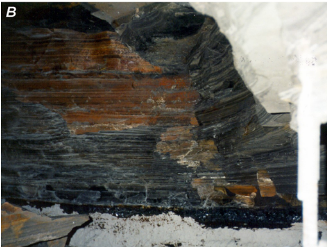
Figure 36.—Roof fall terminating against a large joint face. A, Diagram; B, photograph.
