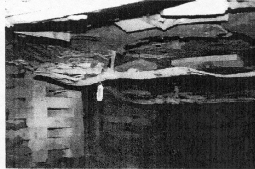
Figure 17. Rear abutment stress damage in L1 entry
