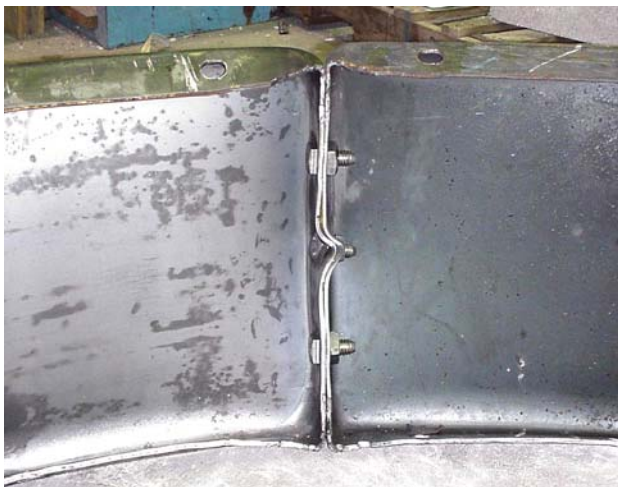
Figure 16. Localized failure occurs near middle bolthole of flange section.
