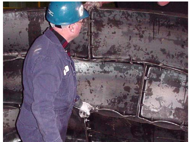
Figure 13. Vertical flange loading causes damage to the flange of the adjacent ring.
