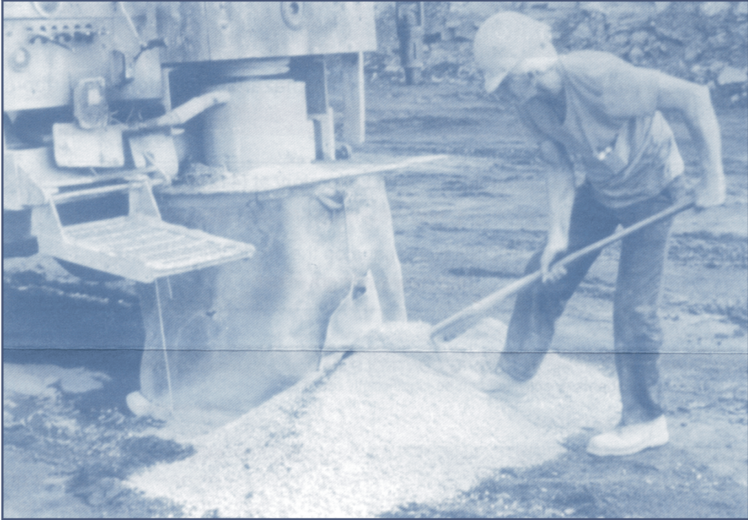
Figure 1. Dry dust collection system for blast hole drill: circular deck shroud.
