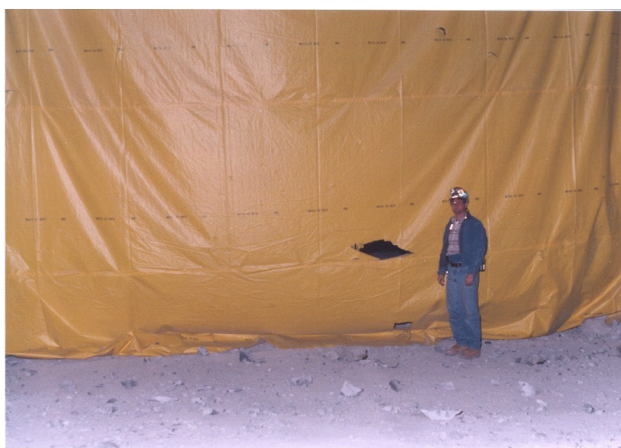
Figure 6. Fly rock damage in brattice cloth.
