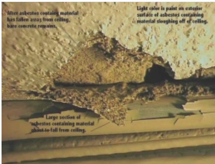
Deteriorating ceiling tiles containing friable asbestos
