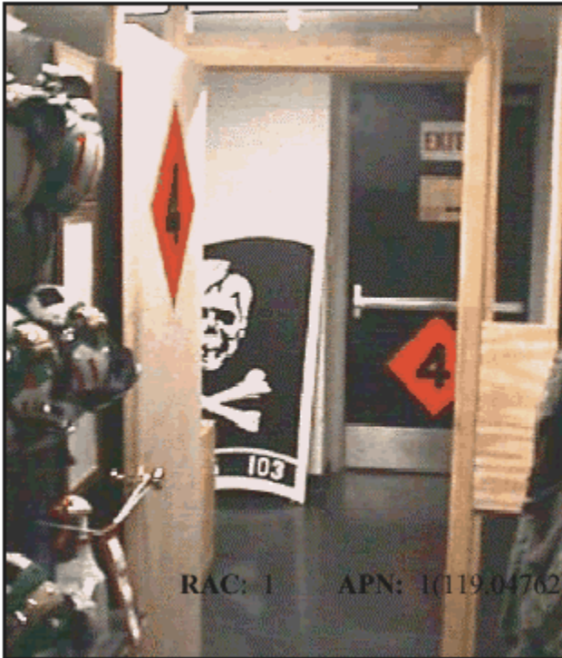
Flight suit storage room exit without emergency egress hardware or NEPA-approved exit signage.
