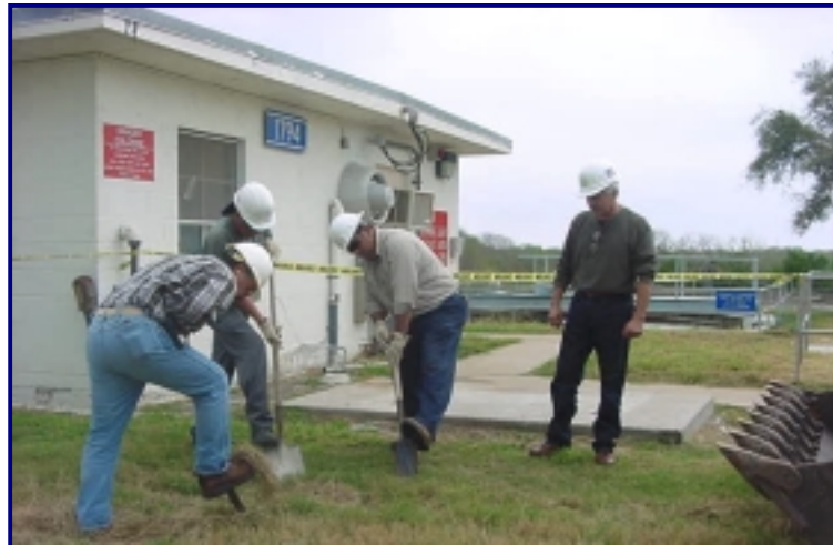
Work crew digs up sewer line for repair at NAS Kingsville as supervisor monitors.
