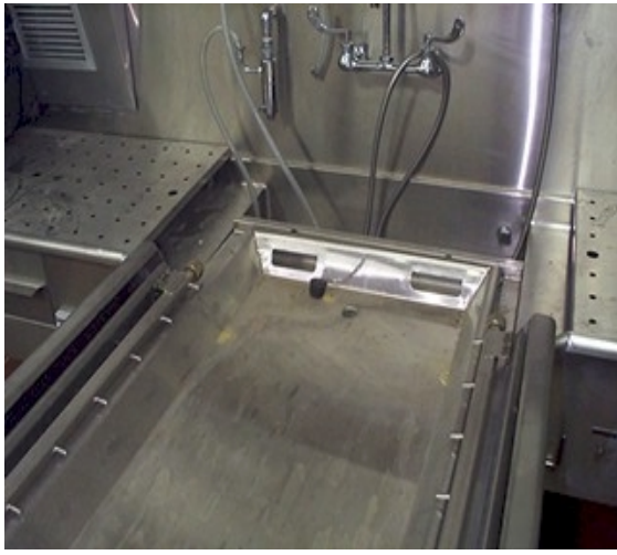
Autopsy table with local exhaust system installed
