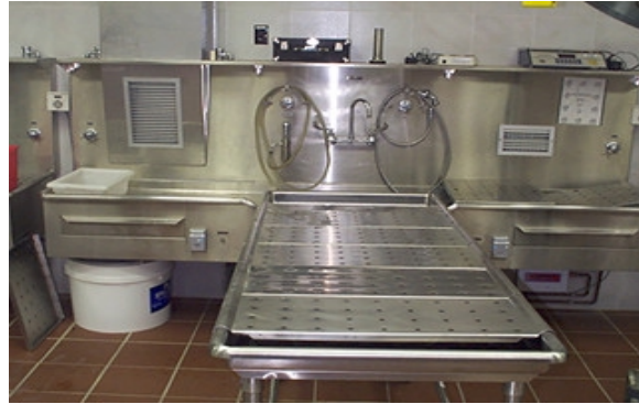
Autopsy table without local exhaust ventilation
