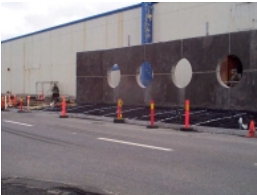
Sidewalks at NEX main store remain free of ice and snow due to the geothermal hot water piping system under them
