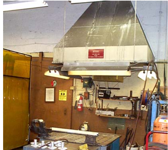
Immovable canopy hood drew welding smoke and fumes directly into the welder's breathing area.
