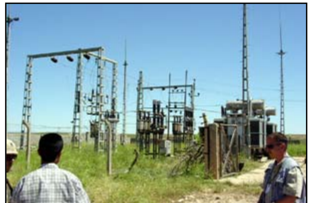
Bechtel assessment team inspects power infrastructure in northern Iraq. (Photo: Bechtel National, Inc.)
