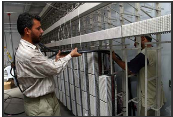
The Al-Mamoun Telephone Exchange where repair work will restore telephone services to approximately 30,000 subscribers. (Photo: Thomas Hartwell)
