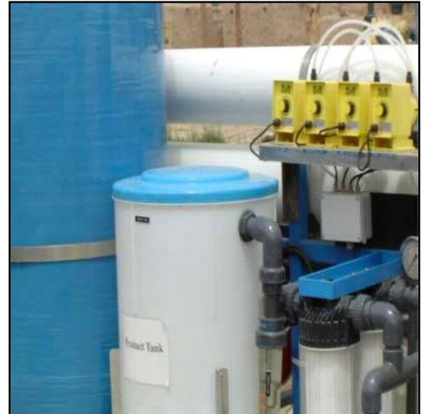
New water equipment at an existing Al Basrah water treatment plant. Photo: USAID
