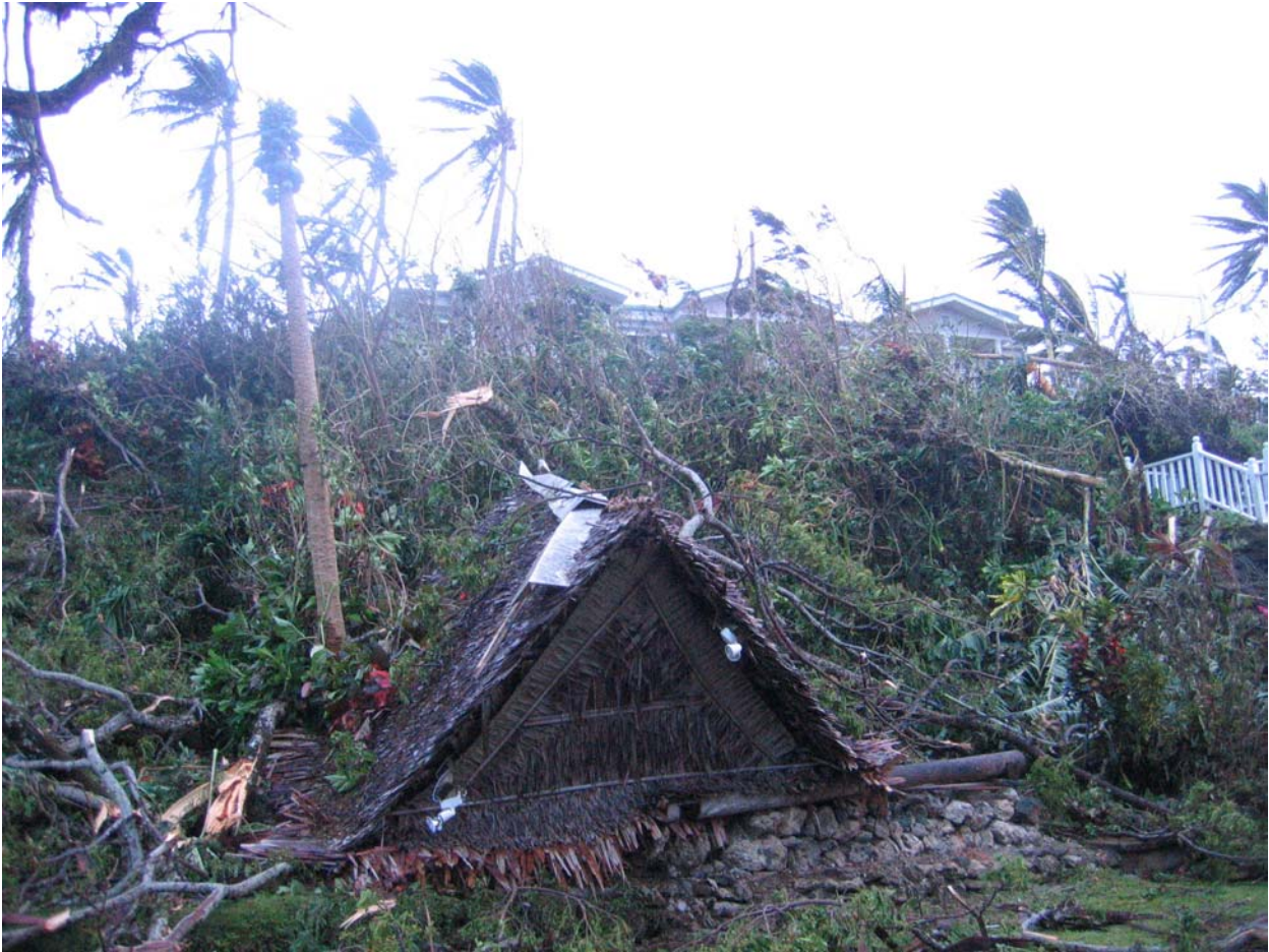
Figure 9. View toward Trader's Ridge Hotel from the main road in Colonia, Yap after Typhoon Sudal.
