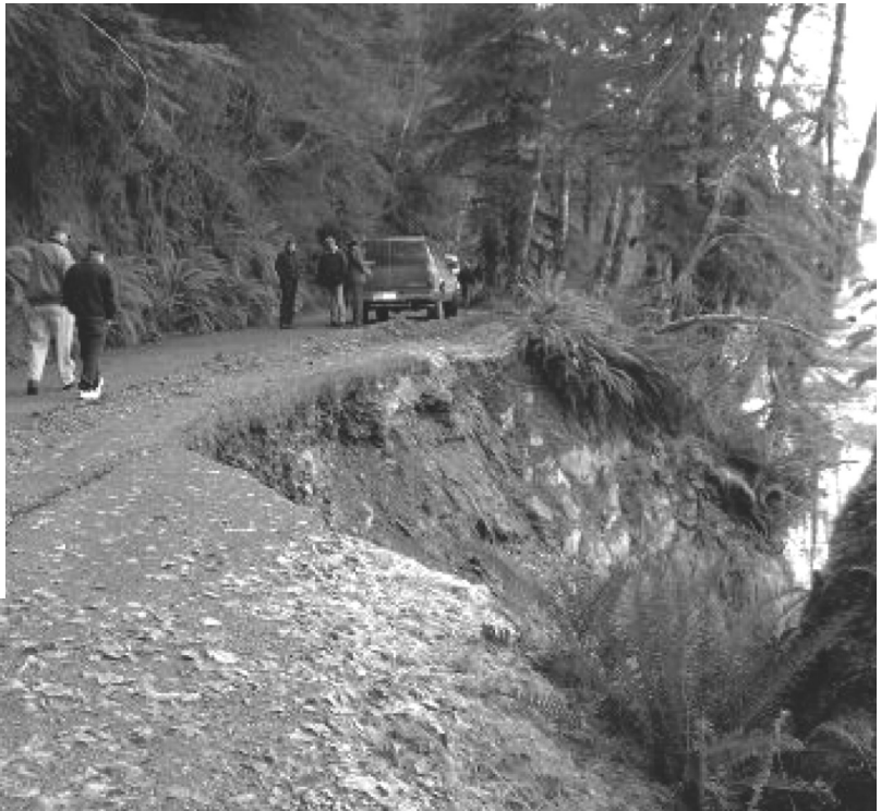
Geomorphological studies provide tribes with alternatives for protecting roads on the Avinalt River, Washington.
