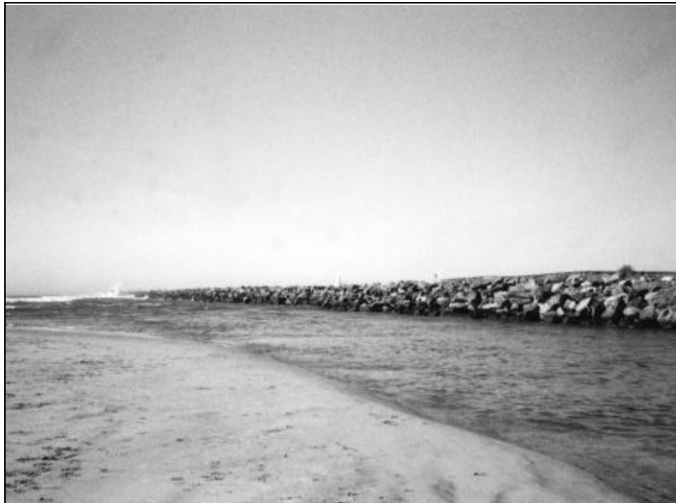
Figure 28. Jetty at the mouth of the San Diego River, California. Such structures, when connected to the upland, form part of the coast line. (Photo by Donna M. Reed)
