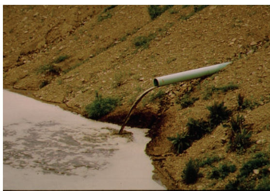
Piped discharges of barnyard and milkhouse wastewater could pollute surface water.
