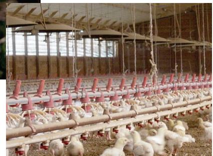
Leaking waterers complicates litter management.
