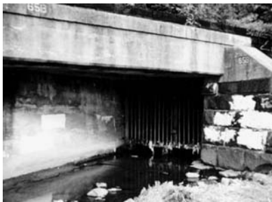
A CSO outfall in Wilmington, Delaware.
