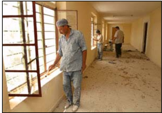
Renovation is almost completed at the Umm Qasr High School for Boys, which was looted and vandalized. (Photo: Thomas Hartwell)
