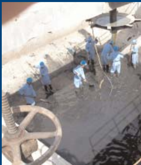
Iraqi workmen cleaning a waste water plant, part of a massive USAID effort to provide clean water and improve health throughout the country.
