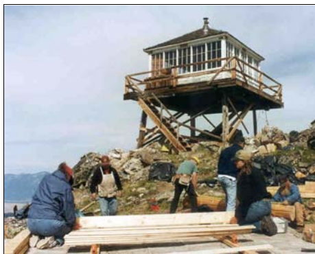
The Bitterroot National Forest in Montana used Fee Demo funds from the Recreation Lodging Program to restore the Gird Point Lookout
