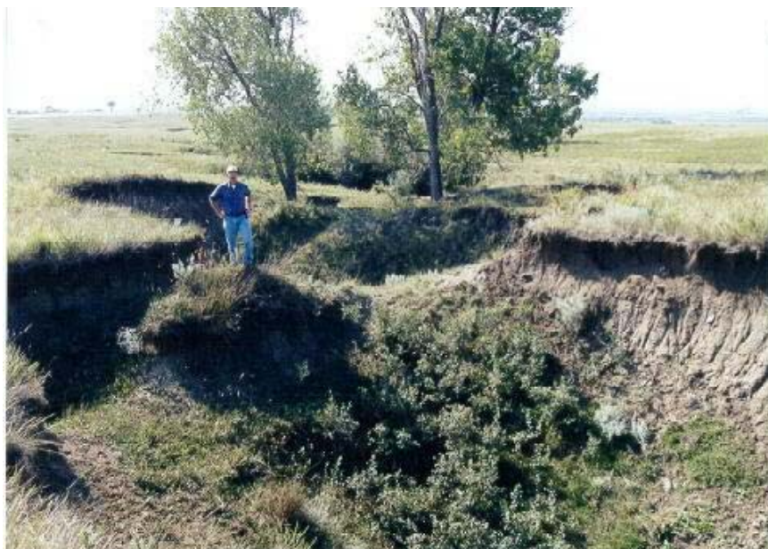
Subsidence features that will not be reclaimed at this time because they are not dangerous to humans or livestock.
