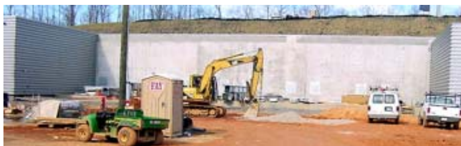
SNS Power Upgrade: The linac tunnel is sized for 9 additional "cryomodules" (top). Augmenting Klystron Gallery is required (bottom).
