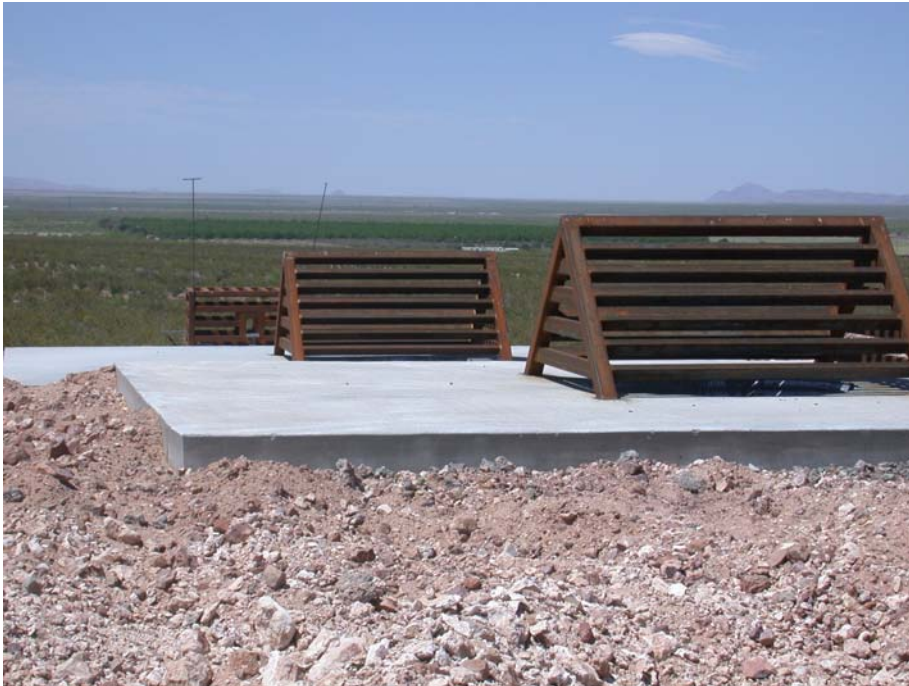
Bat Cupolas and Concrete Covers over Vertical Openings at Spar Group Project.
