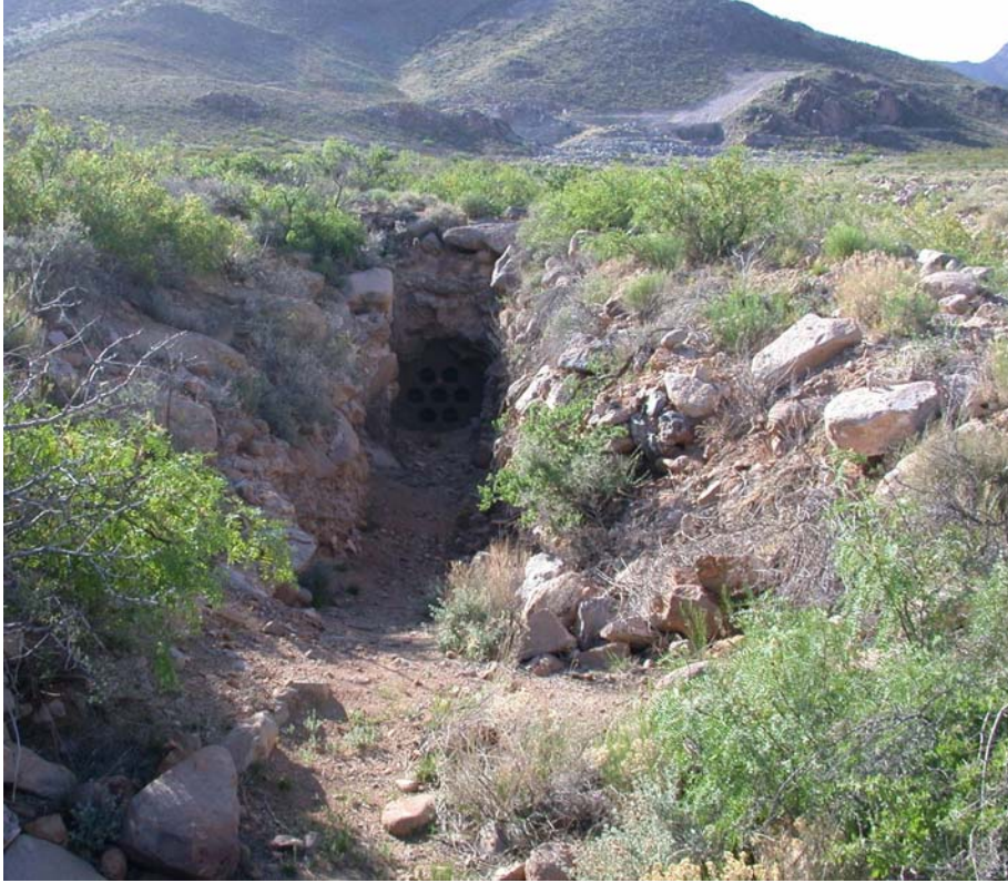
Pipe Array Drainage for Under Ground Workings at Stevenson Bennett Mine Project.
