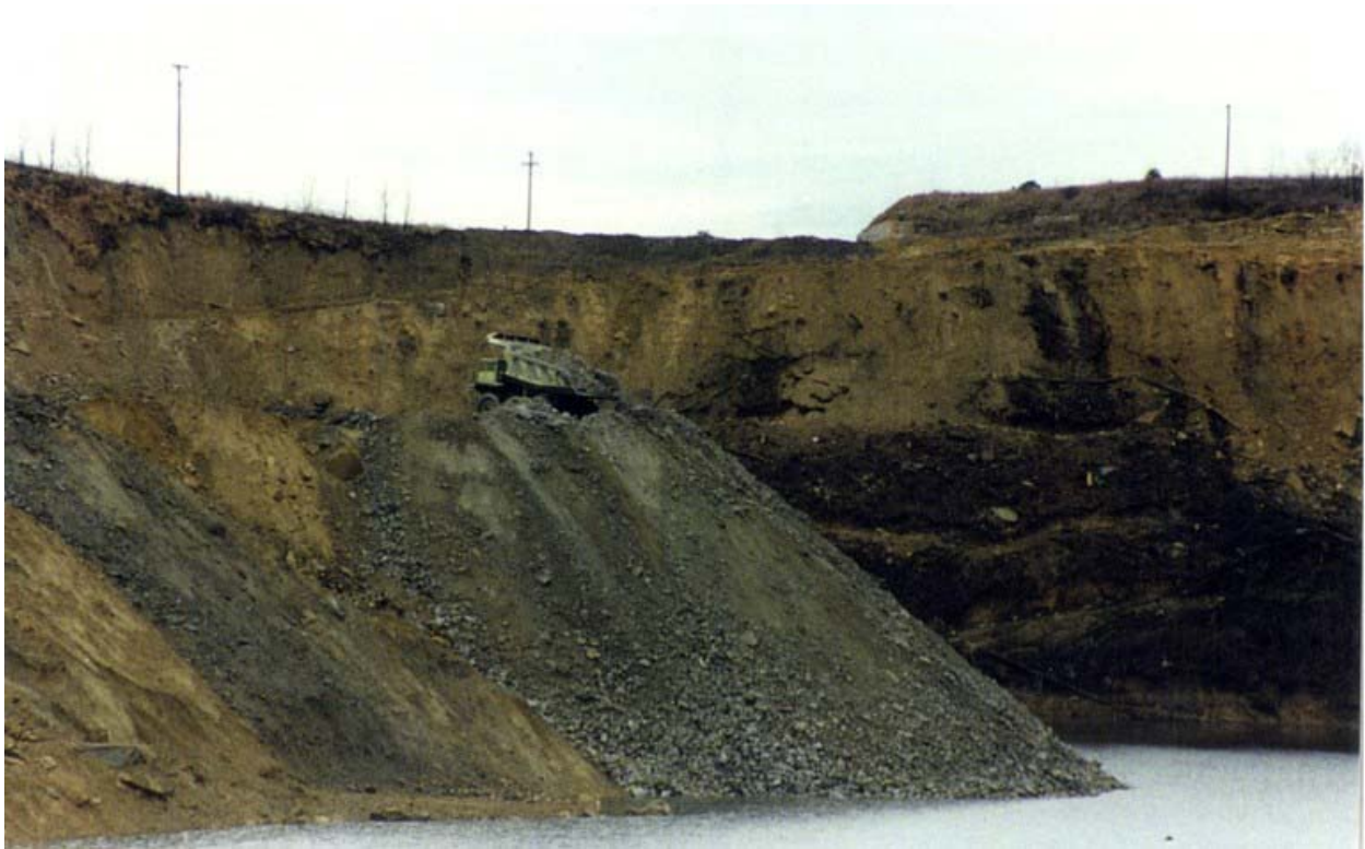
Photo 10. Construction of Seepage Barrier (End Dumping by Rock Truck) - March 6, 1995. Source: GAI. The work is being conducted at the southwest side of the impoundment.
