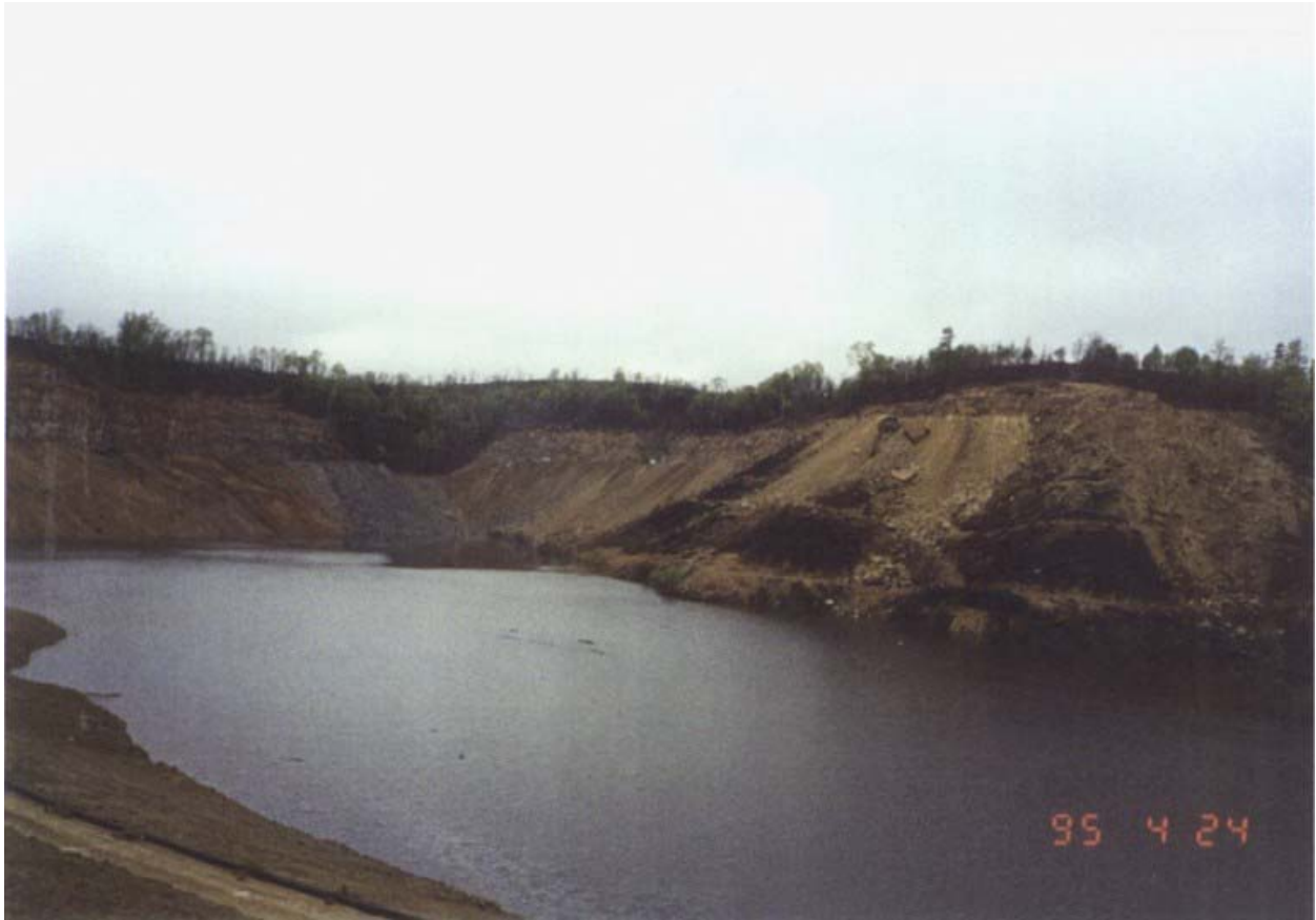
Photo 12. Seepage Barrier by 2000 Breakthrough (During Construction) - April 24, 1995. Source: GAI. The 2000 breakthrough area is located at the left-center of the photo. Pool elevation 1,000 feet msl. Mine roof elevation 973 feet msl.
