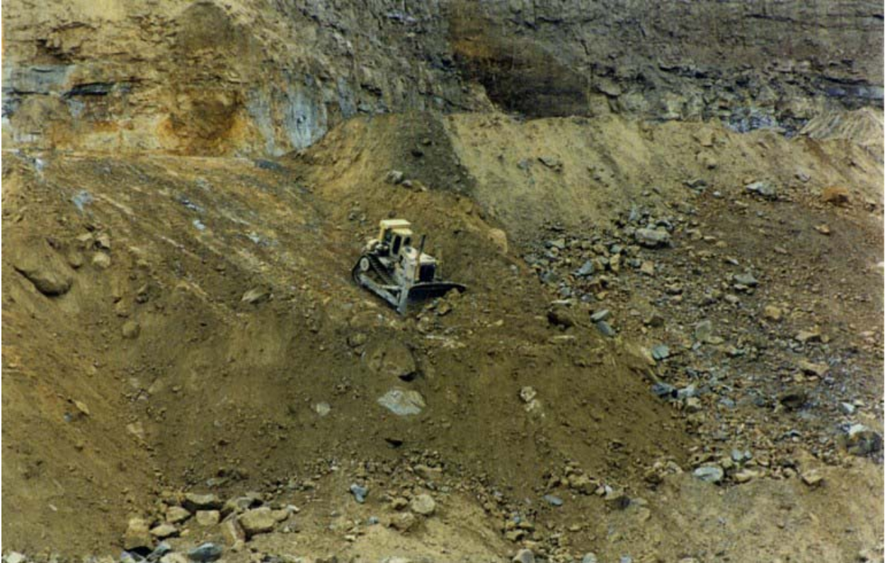
Photo 9. Construction of Seepage Barrier (Dozer Work) - March 6, 1995. Source: GAI. The work is being conducted at the southwest side of the impoundment.
