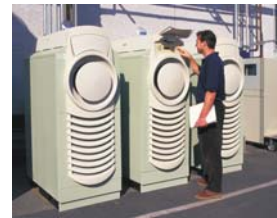
Three 30 kW Microturbines running on LFG in CA
