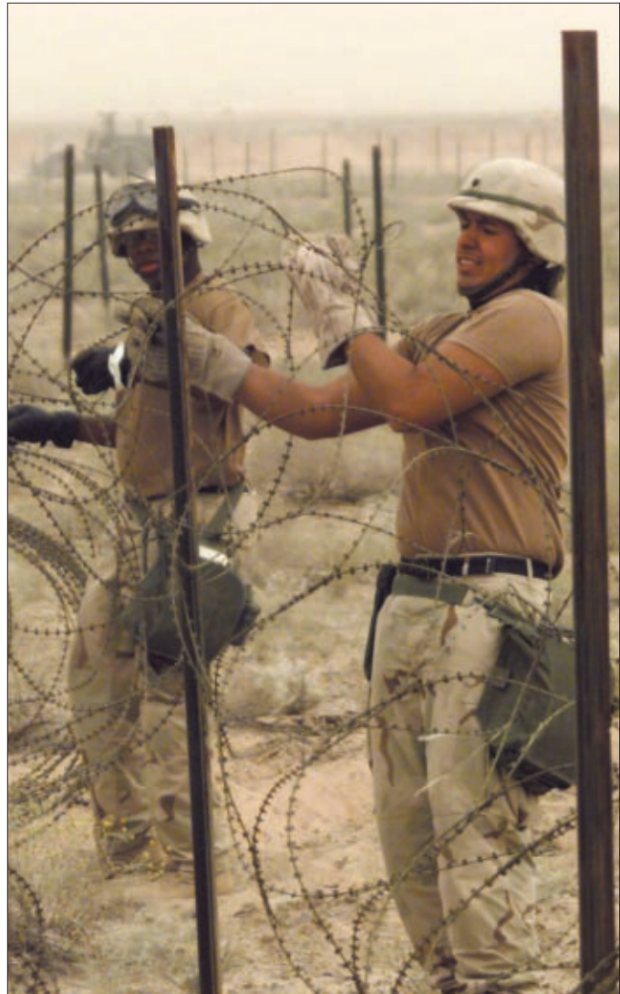
Spec. Jose Lopez, a sheriff’s deputy in Broward County, Fla., and a colleague put up some concertina wire along a yet-to-be-built fence line as Army Reserve soldiers with the 724th Military Police Battalion find themselves pitching in to build the new EPW facility they will be guarding.
