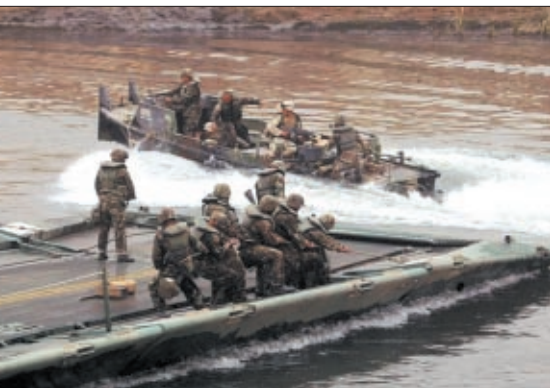
Members of the 459th Multi-Role Bridge Company construct a floating bridge over the Tigris River on the outskirts of Baghdad.
