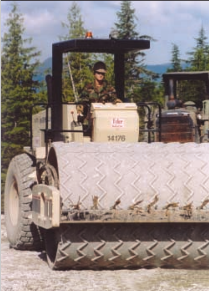
Army Reserve Pfc. Ashlee Ohlfs operates the vibe roller, a steamroller-like flattening machine on the under-construction road to Metlakatla on Annette Island, Alaska.
