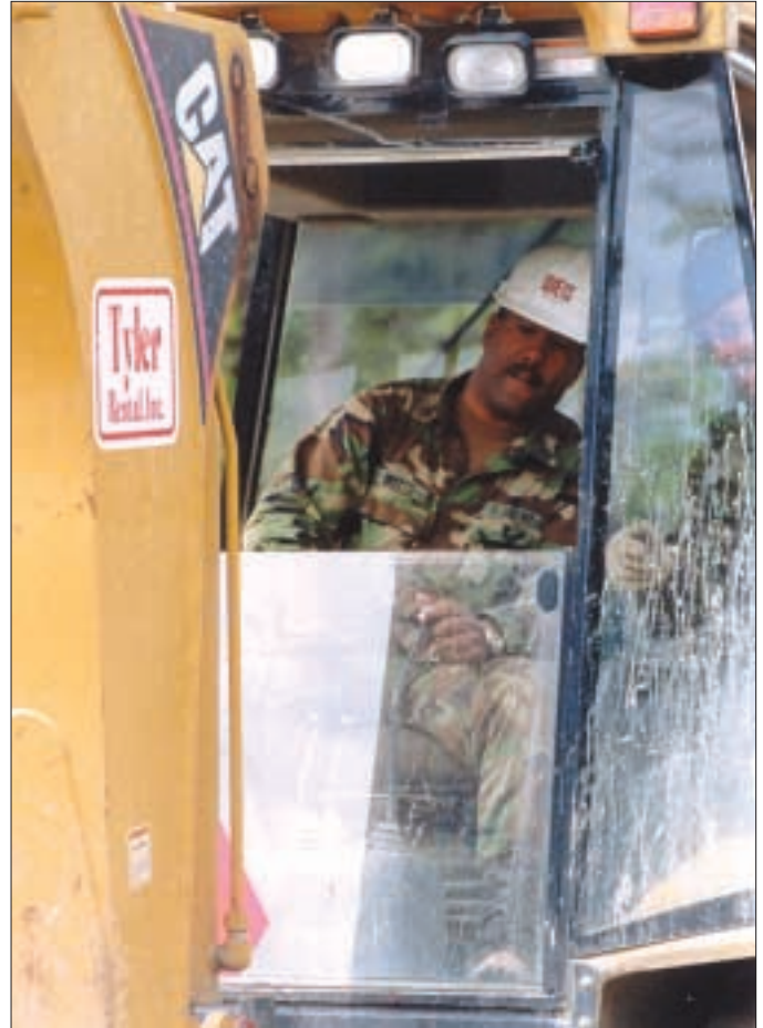
Army Reserve Staff Sgt. 1st Class Maurice Britts with the 367th Engineer Battalion operates an excavator on an Alaskan road during Operation Alaskan Road.
