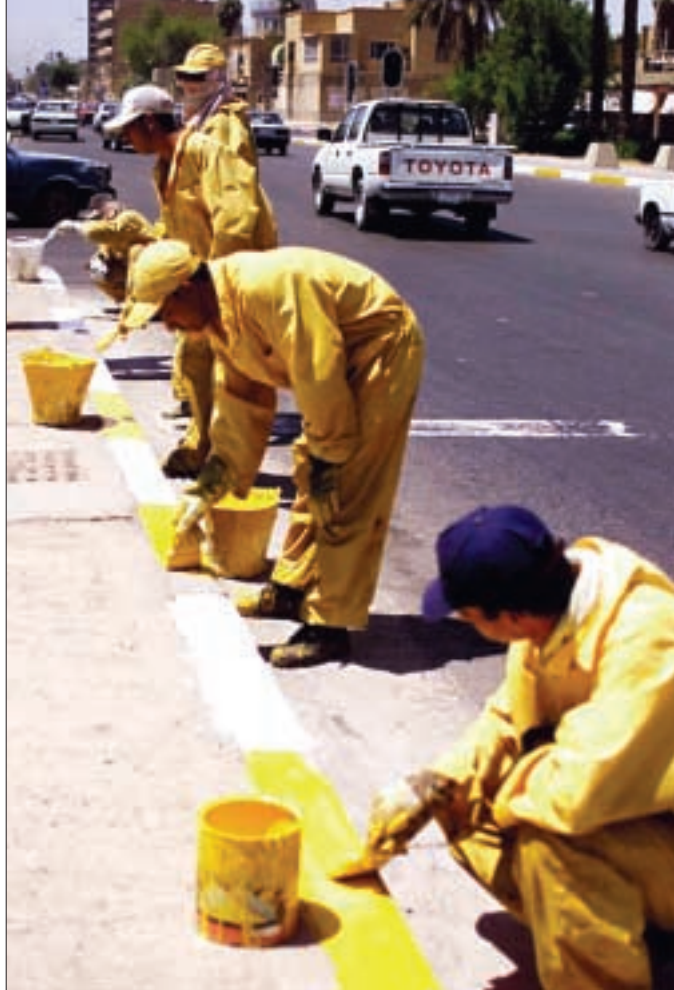
Iraqi road workers lay down a few coats of paint on a downtown curb as part of Baghdad's road restoration efforts.
