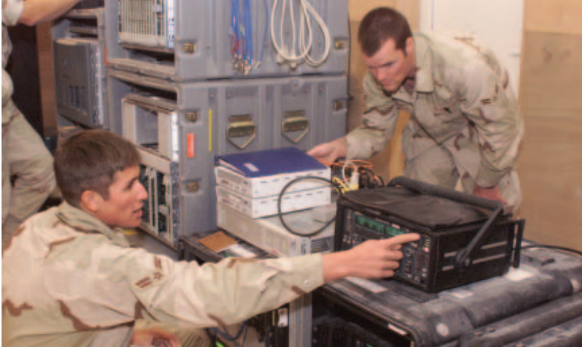
Communications professionals test the fiber optic link in the new communications network control center while deployed in support of Operation ENDURING FREEDOM.
