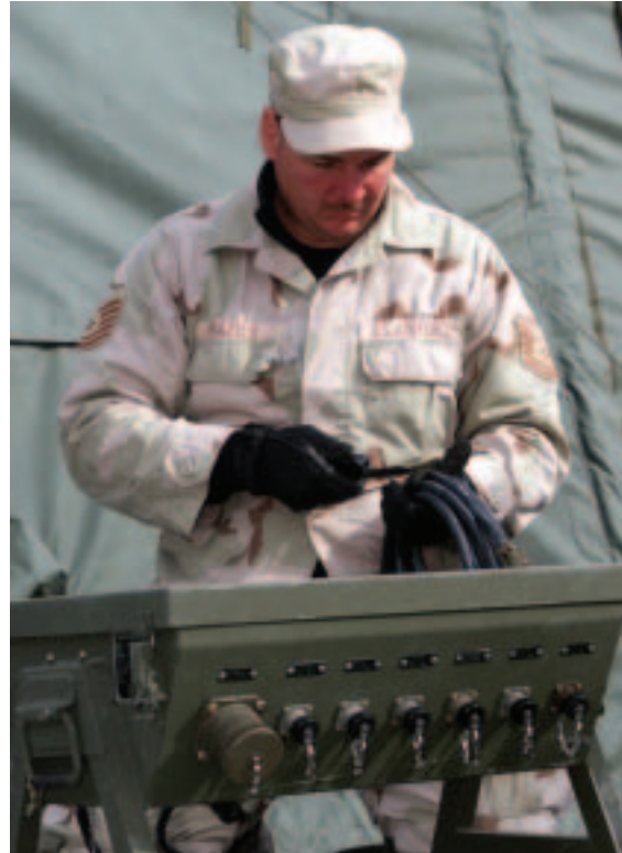
TSgt Todd Frazier, a 376th Air Expeditionary Wing, Civil Engineering Squadron electrician, sets up an electrical distribution box designed to provide 110 volts of power to outlets at a deployed site in Kyrgyzstan.
