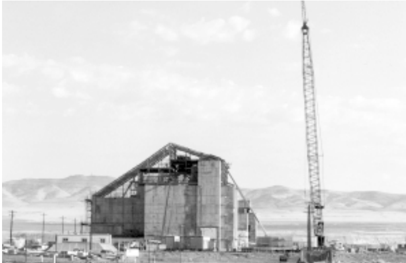
Placing a 75-year roof over the remaining portions of DR Reactor was the last step in the cocooning process.
